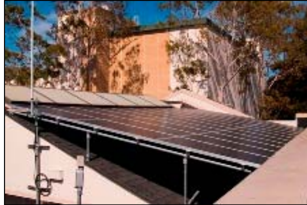
Solar panels on the Utilities Administration building
