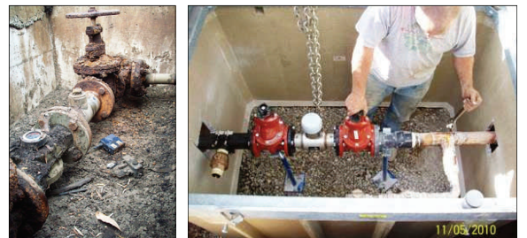
Infrastructure Equipment - Before and After
